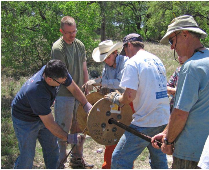
Several people were required to unspool the new cable. Bobby DeVos photo
